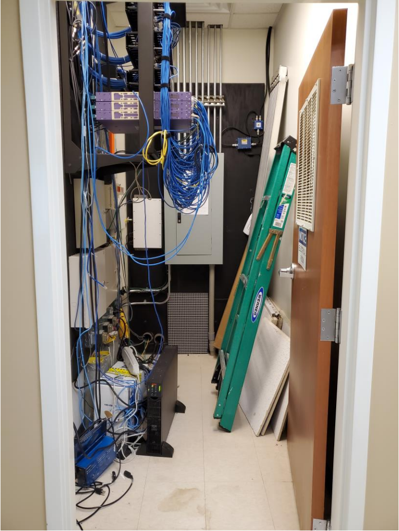
Inside Server Room
