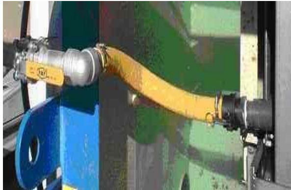
Figure 29 - Typical field installation of blower air line
