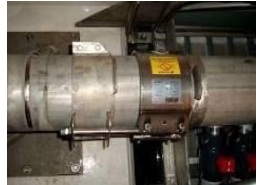
Figure 31 - Typical field installation of the permeate line
