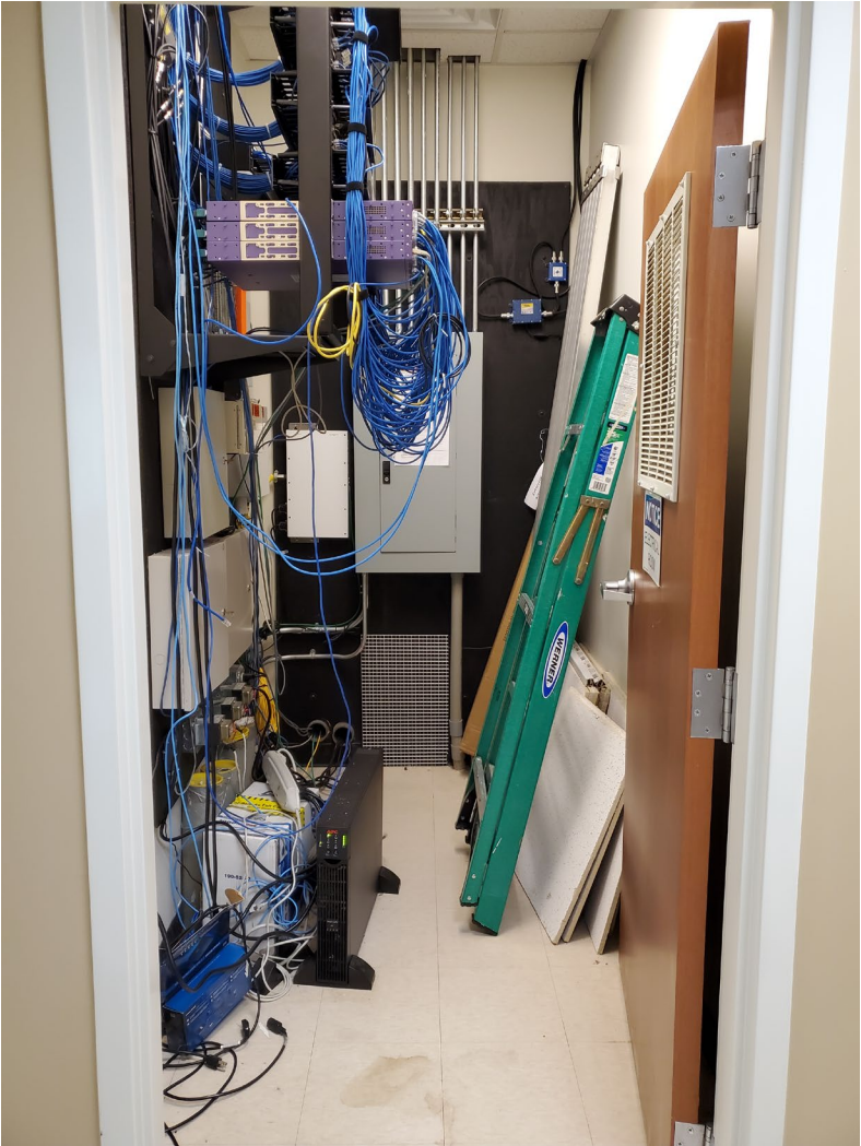
Inside Server Room
